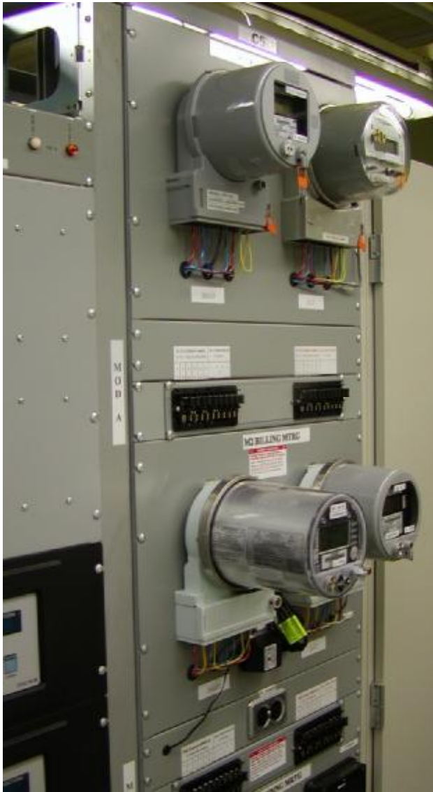
Front Face of Relay Rack
